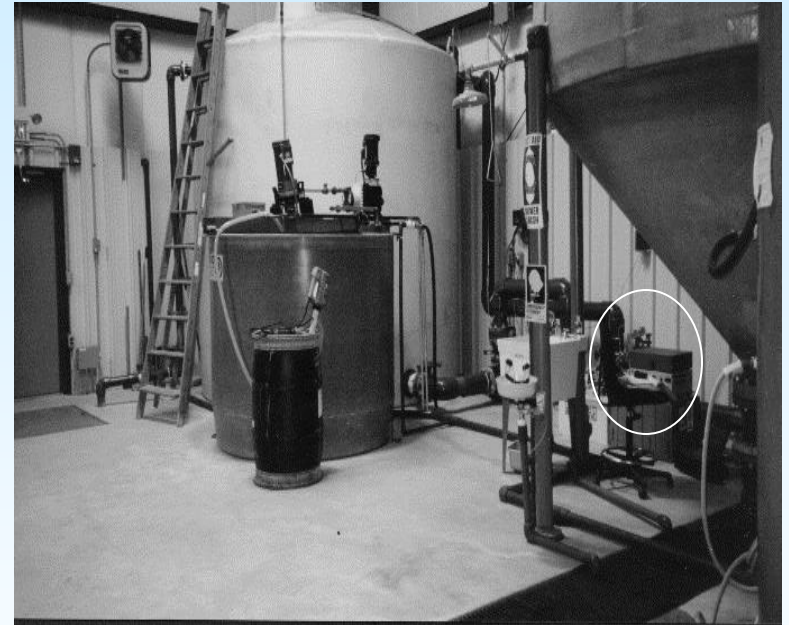
A groundwater treatment facility at the Naval and Engineering Station in Lakehurst, NJ, where the field study was conducted.
